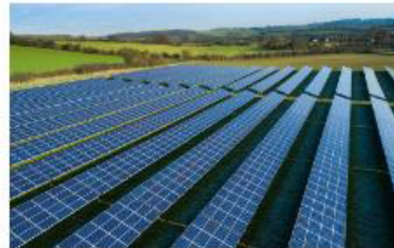
Solar power plant. Source: JBM Solar.
